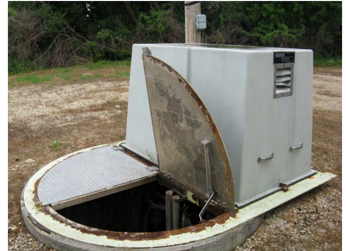
Lift station wetwell/valving
