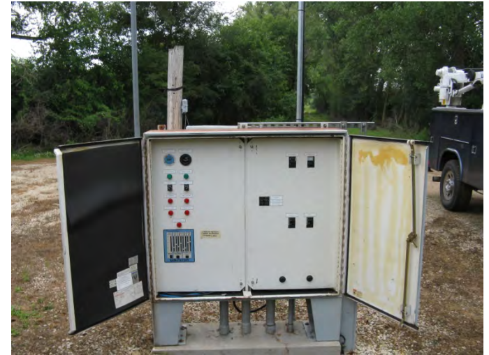
Lift station controls
