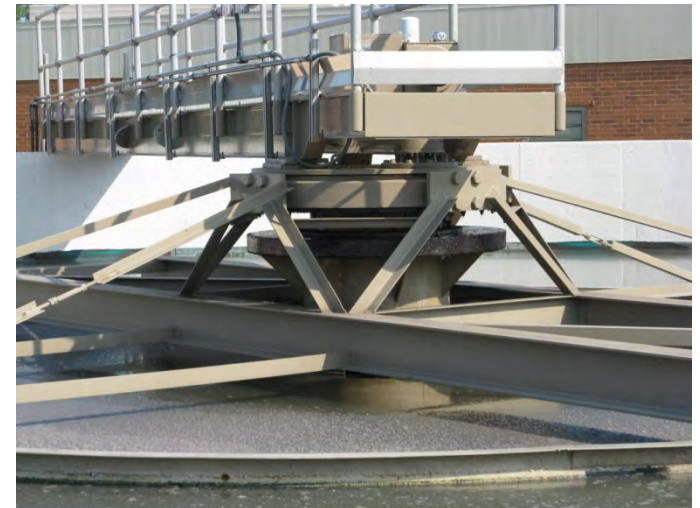
Clarifier bearing assembly
