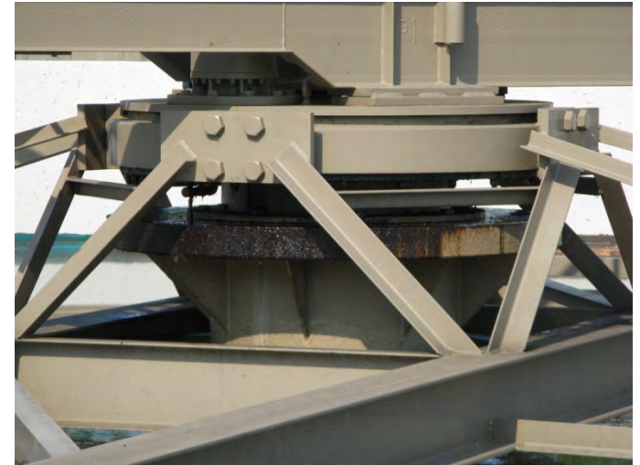
Leaking clarifier bearings
