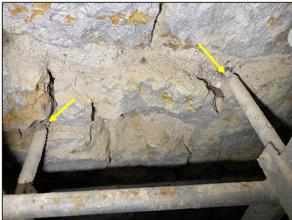
Photo 37: Corroded ladder connections at wall
