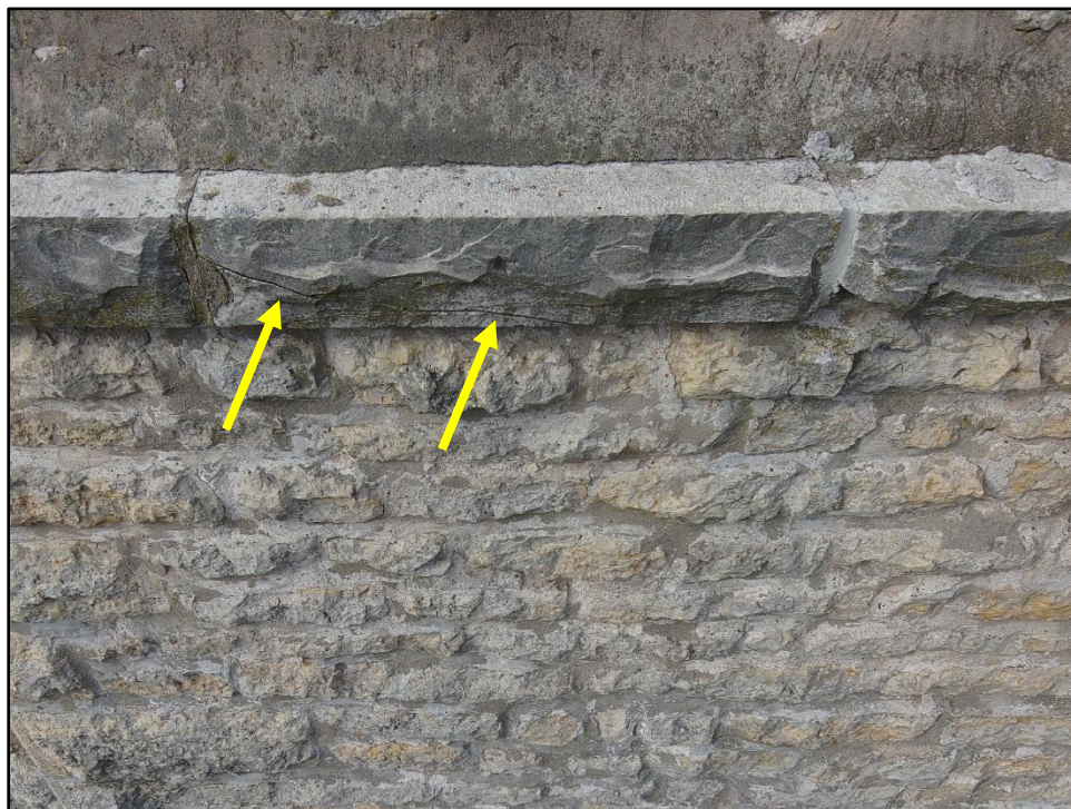
Photo 13: Horizontal cracks in stone
