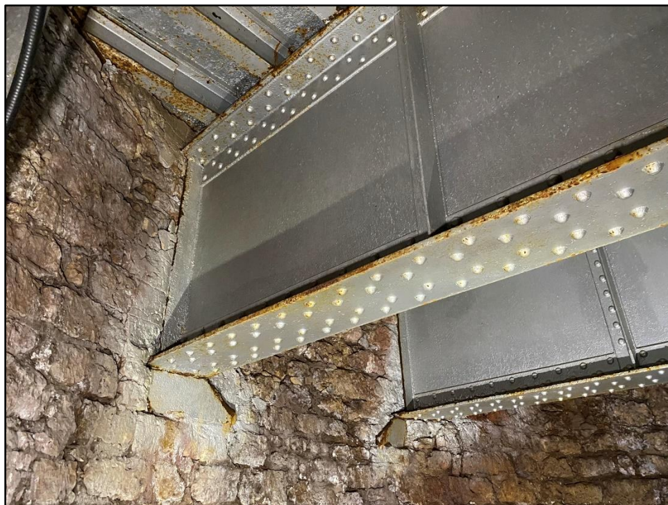
Photo 31: General light corrosion on support structure
